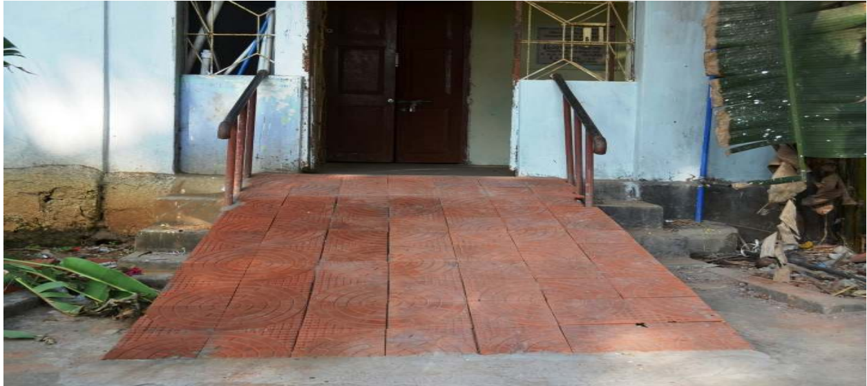
Ongoing construction of Ramp at Prema Samaajam (a home for elderly persons), Vizianagaram
